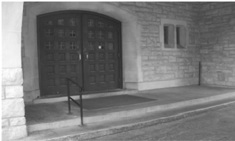
This is the northwest entrance to the church, under the portico. When this area is renovated for accessibility, individuals can be dropped off under the existing covered driveway, but will no longer have to climb three steps to get inside the church.
